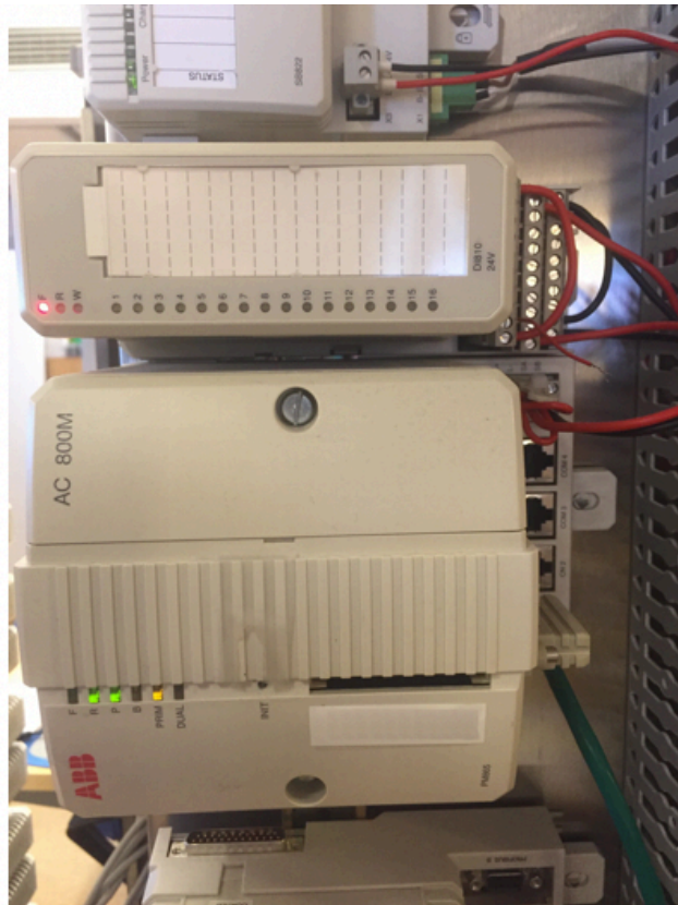
Running Bloqqi on controller hardware (ABB AC800M)
