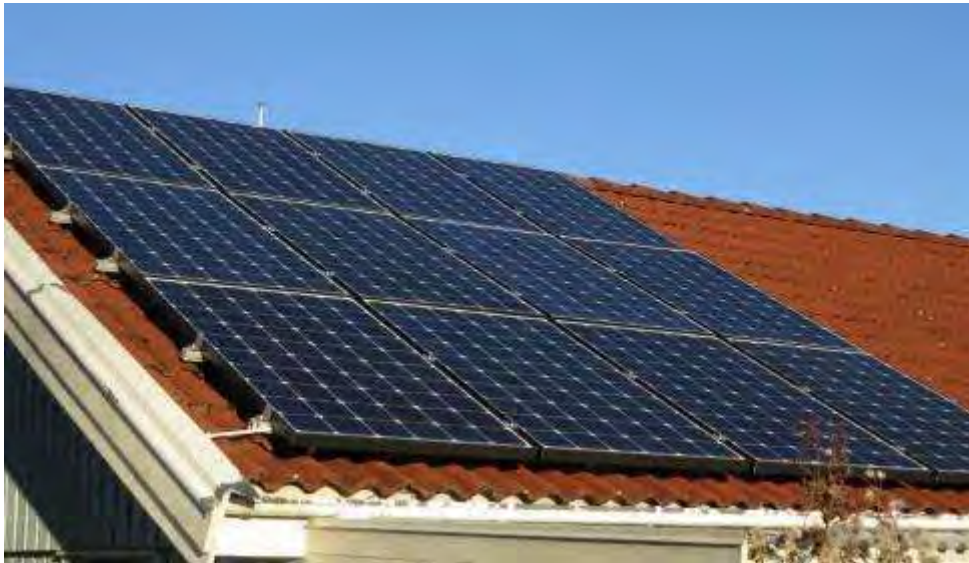
20 sqm solar panels on garage roof, Nov 2012 Generated 2700 W at noon March 10, 2013
